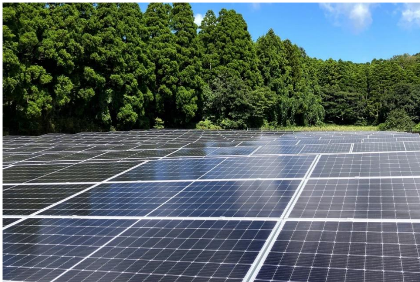
Solar Power Generation Facilities Engaged in Virtual PPA.
