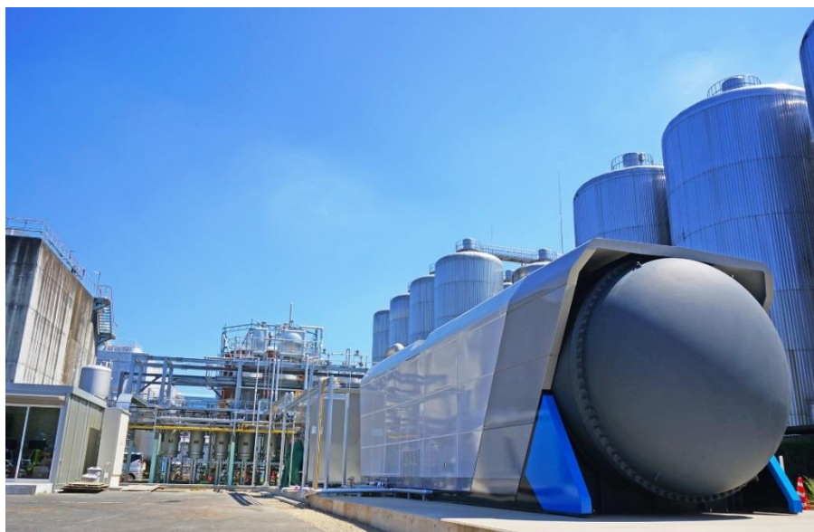
Facility at the Asahi Breweries Ibaraki Brewery (Left rear: Brewery wastewater treatment facility; Center: Biogas refining equipment; Right front: SOFC)
